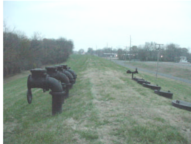
20. Pipes on levee along 6 th Street between Route 45 and downtown.
