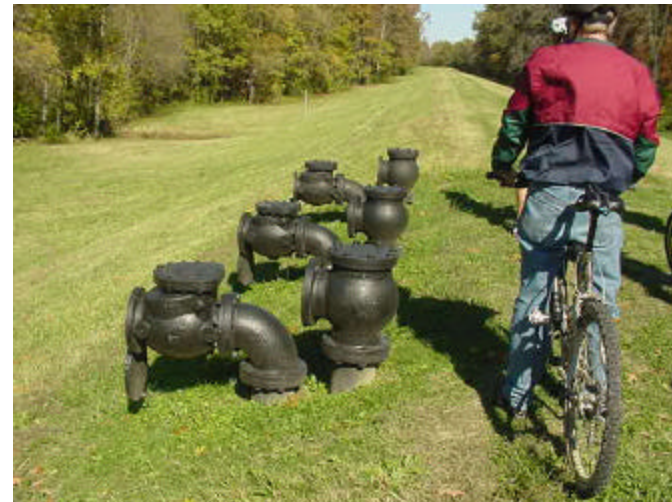
8. Typical pipes at pump station.
