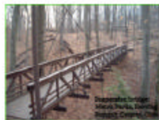
Suspension Bridge A suspension bridge is proposed to cross Parkins Creek. Coverage of this nature preserve flows through to sensitive fish and wildlife species and offer an excellent situation for park visitors.
