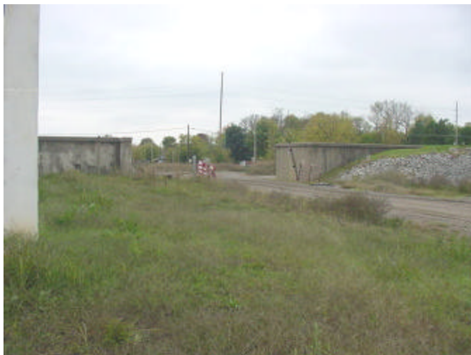
23. End of earth levee and beginning of floodwall west of Convention Center at Campbell Street.
